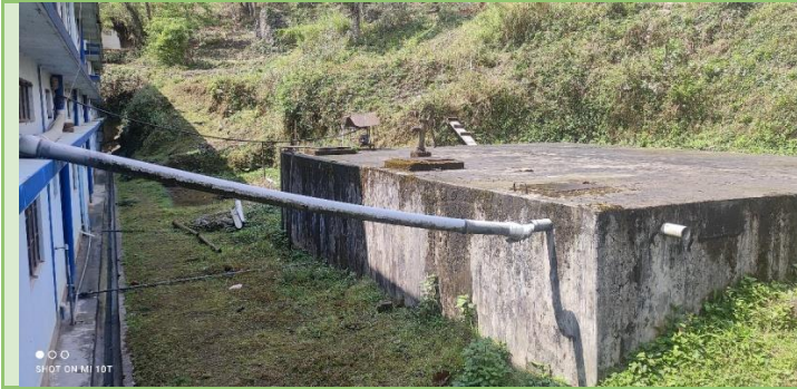
Rain Water Harvesting at SJC Girl's Hostel
