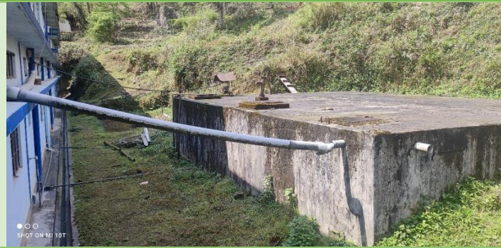
Rain Water Harvesting at SJC Girl's Hostel
